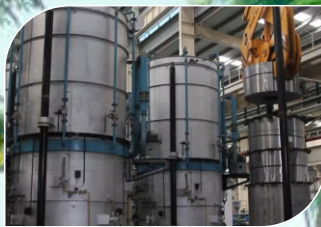
Seco Warwick Batch Annealing Furnace (Poland)
