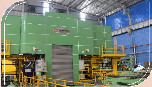
Cold Rolling Mill
