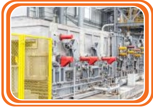
ELECTROLYTIC CLEANING LINE
